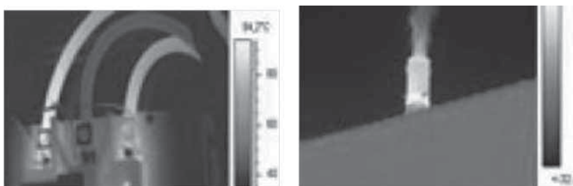
Figure 7. Thermograms of electrical installations and a chimney
