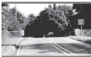
Fig. 6: Application of markings in the form dragon teeth on the carriageway surface
